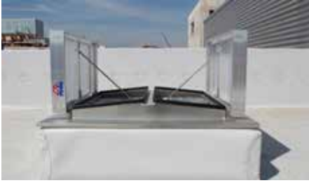
Single unit on base on an industrial roof
